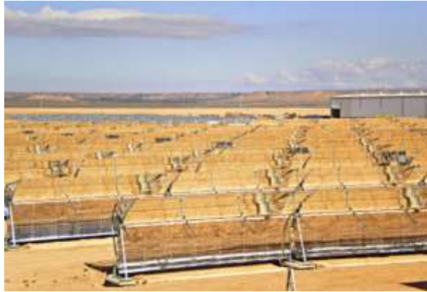
Figure 16: Ain Beni Mathar, Morocco: hybrid solar (CSP)-natural gas plant
